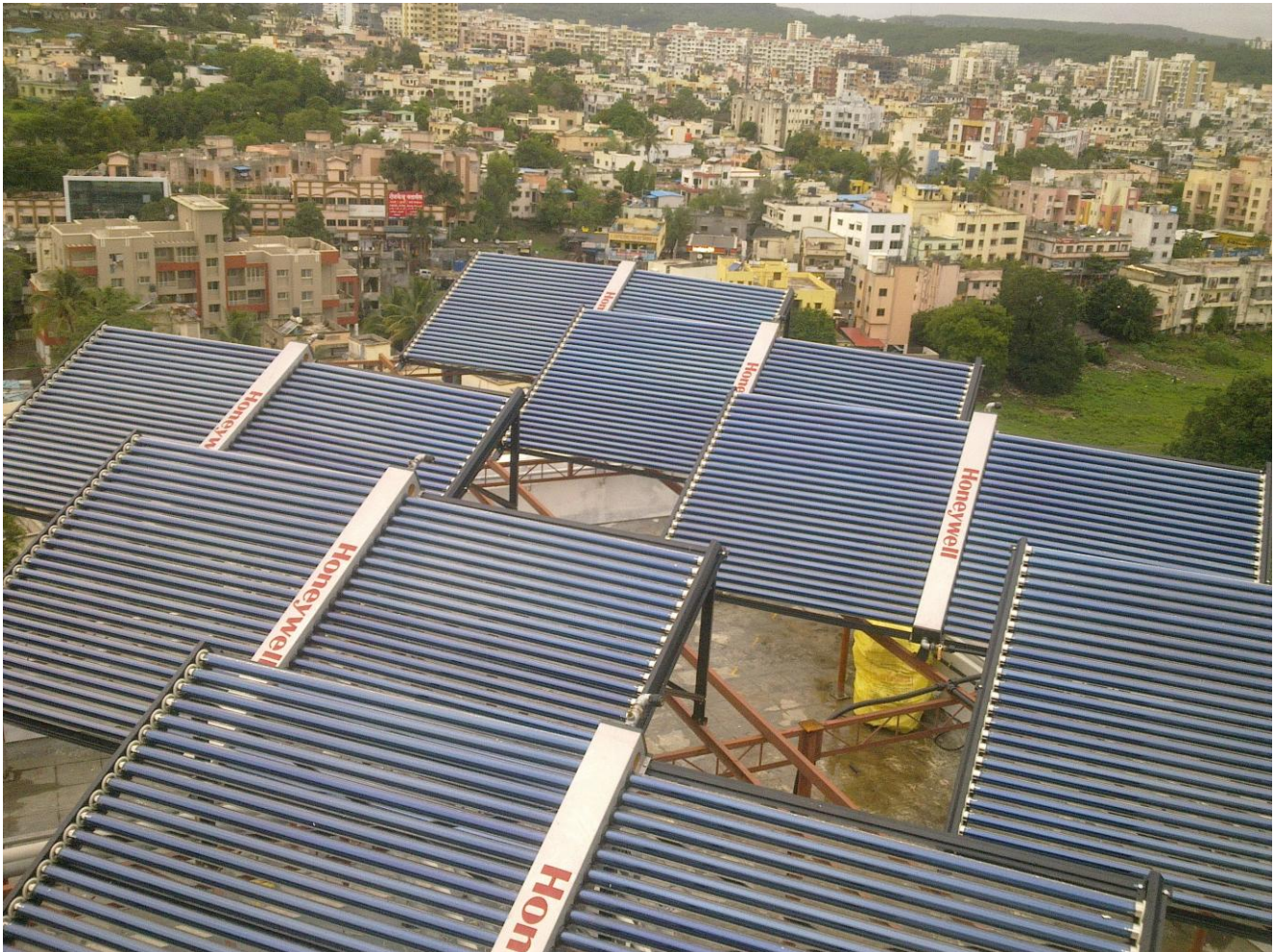
20000 LPD Solar Water Heating System
